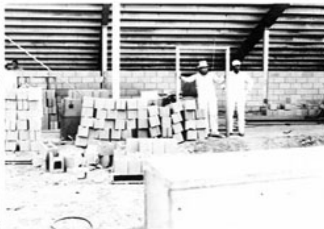
Something new?? A dressing room for the football players is well underway!
